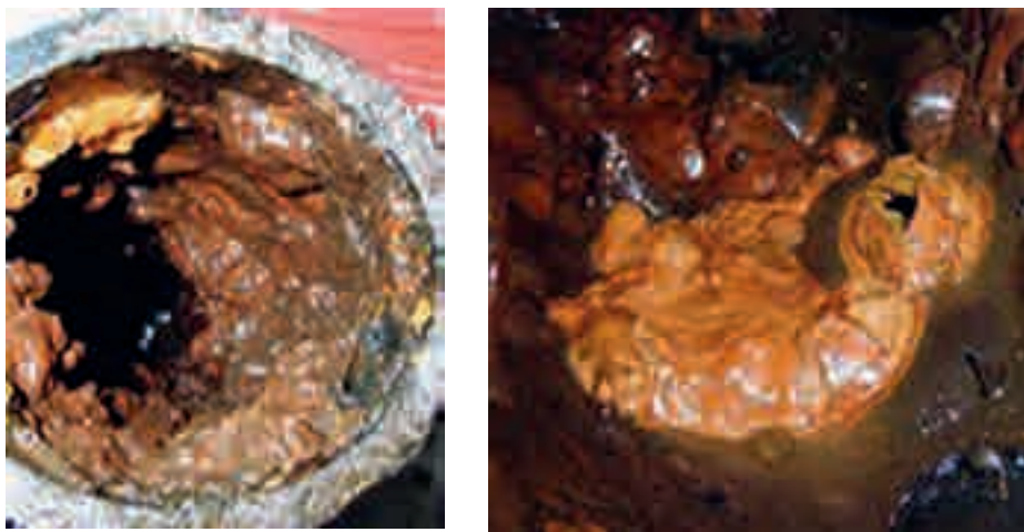
Fig. 4: interior of a drinking water pipe. Kindly authorized by Prof. Flemming, IWW Water Centre, Mülheim an der Ruhr, 2012
